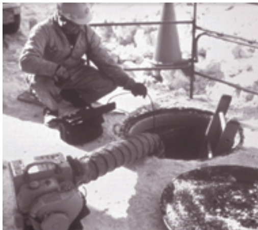
Continuous ventilation and testing are critical in any confined space with a harmful atmosphere.
