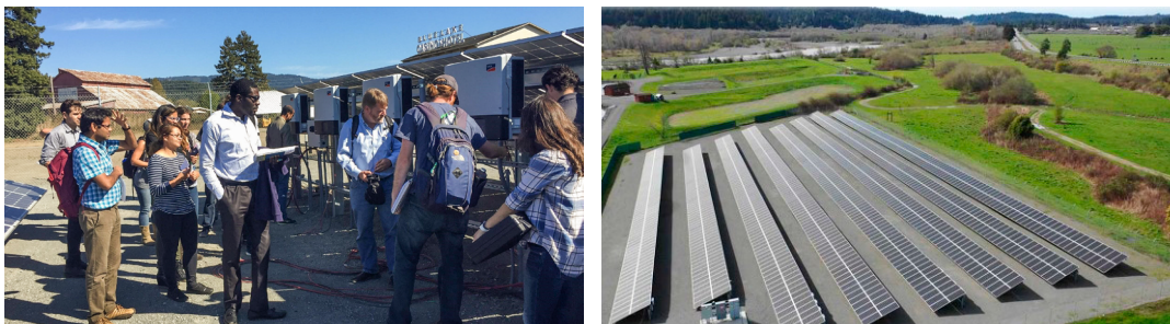
Left: HSU students onsite at BLR investigating the community scale microgrid solar array and inverters. Right: Aerial view of the 420-kilowatt solar photovoltaic array at BLR, with CA Highway 299 and the Mad River in the background.
